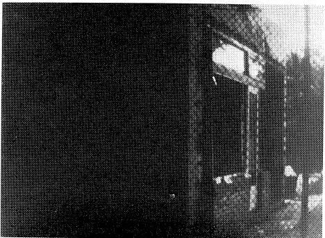
d. condition after the explosion
