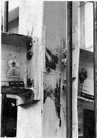
Fig. 6.16a. Plastic deformations of a beam-to-column connection designed with formula (3-35) and/or (3-36).
