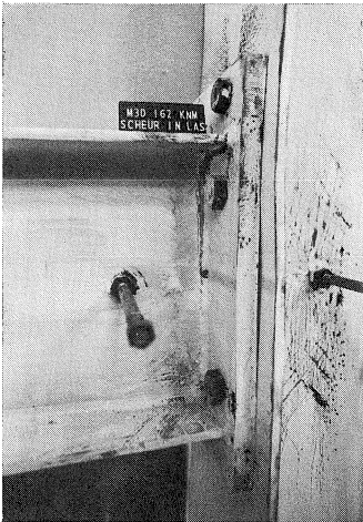
Fig. 6.13a. Plastic deformations of a beam-to-column connection designed with formula (3-35) and/or (3-36).
