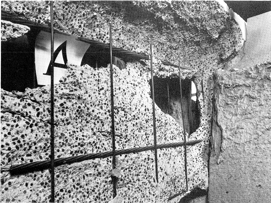
Fig. 31. Beam b_1 after the fire test.
