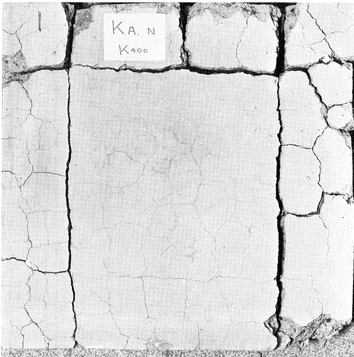
Fig. 41. Slab in series c after the fire test.
