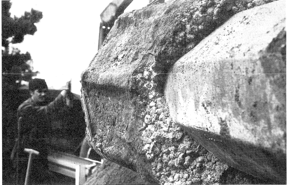
Fig. 11. Photograph of deteriorated lamp post.
