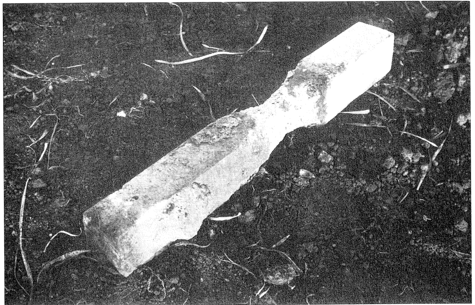
Fig. 9. Deteriorated greenhouse foundation pile (12).
