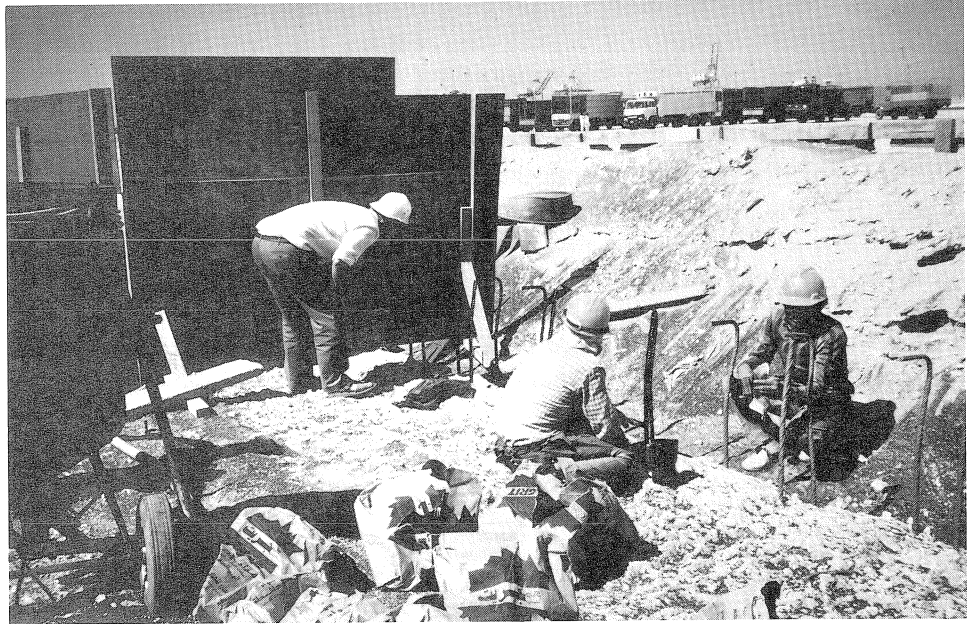
Fig. 42. Photograph of the coating operation of steel reinforcement during the repair of the Al-Shindagah Tunnel in Dubai.
