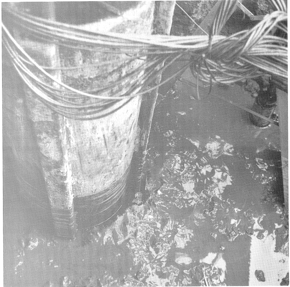
Fig. 7.11 Picture of the gap behind the pile, after the test.
