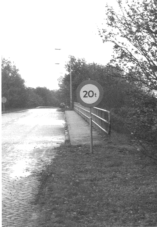
Figure 1. Load limitation to 20 tonsting on a viaduct due to a reduction of the load-bearing capacity from ASR
