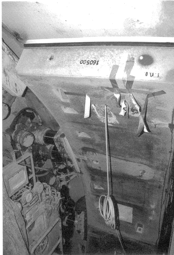
Figure 14. Assembly of one of the segments of the structural monitoring ring in the Botlek railway tunnel. The cable of the data acquisition system is connected to the junction box in the segment to provide monitoring data during ring assembly.
