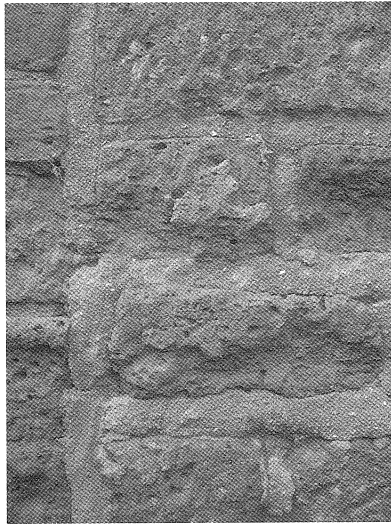
Fig. 13. Spalling of Römer tuff, church tower at Tienhoven.
