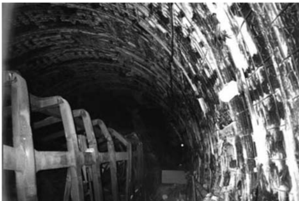
Figure 1. Fire damage in Channel tunnel
