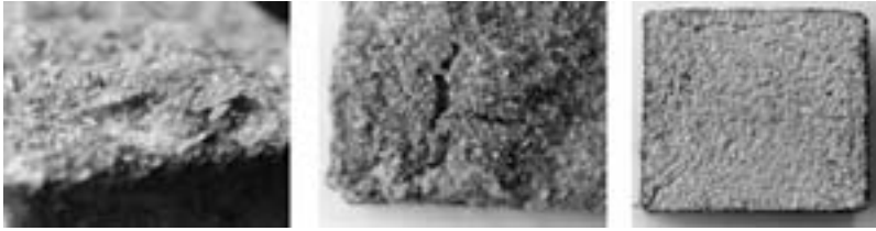
Figure 7: Peeling of paint (left), bulging, cracks, efflorescence (middle), cracks (right)
