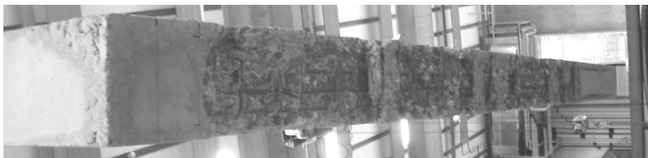
Figure 34: Internal steel reinforcement is clearly visible after concrete cover rip-off
