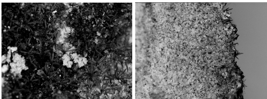
Figure 10. Details of biogenic layer on sample 8 and disintegration of the limestone (right picture)
