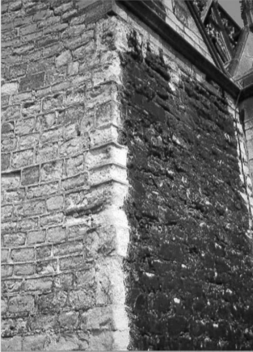
Figure 16: South façade transept. Consequence of use of incompatible re-pointing: damage to Lede stone – situation 1991. (photo: Rob van Hees)
