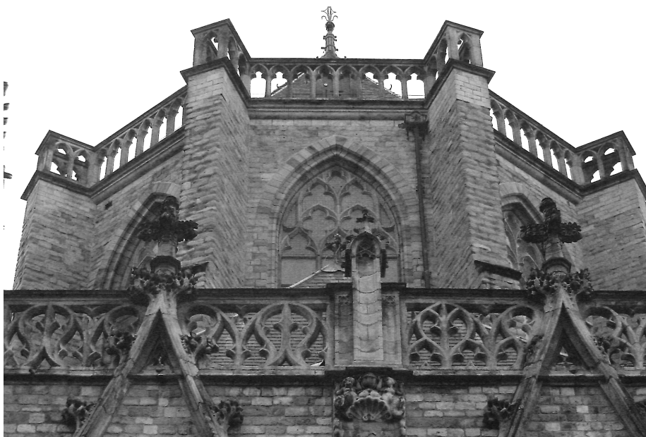
Figure 10: View on the high windows of the choir in Obernkirchen sandstone (photo: author, december 2005)
