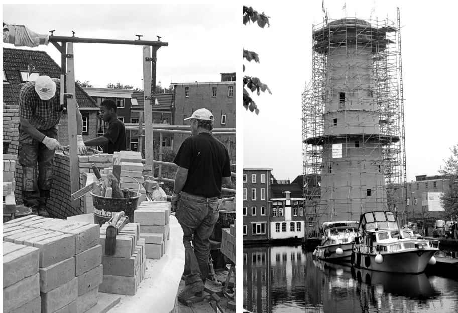
Figure 9. Construction of the windmill "de Kameel" (the Camel) in Schiedam in solid masonry (2009). For the choice of brick and bedding mortar the determining factors were good water tightness and good deformability (low E-modulus) of the wall masonry.
