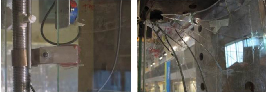
Figure 10: Seized second highest sliding sleeve and locally cracked glass pane
