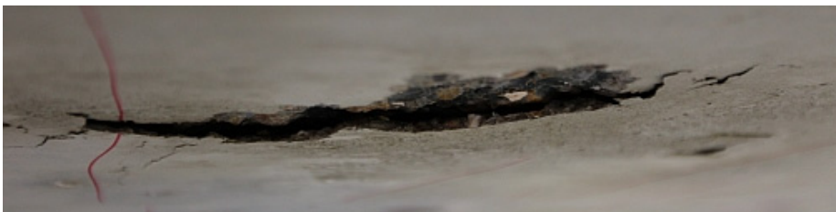
Figure 8. Punching damage at the bottom of a slab after an experiment
