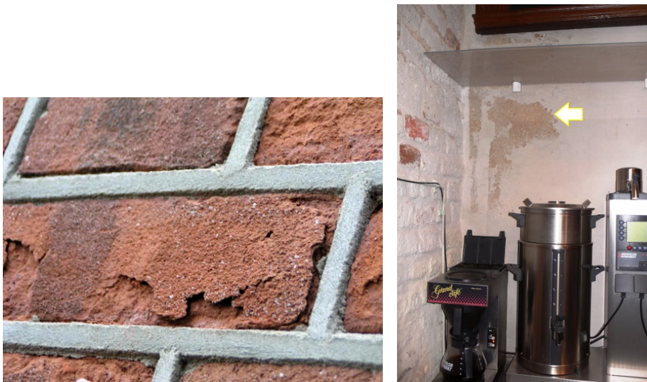
Figure 7. Left: Spalling of brick caused by salt crystallisation (Netherlands). The brickwork had been treated with a water repellent: concentration of salts and crystallisation-dissolution cycling under the water repellent layer. Right: Sanding of surface layer of plaster caused by salts.
