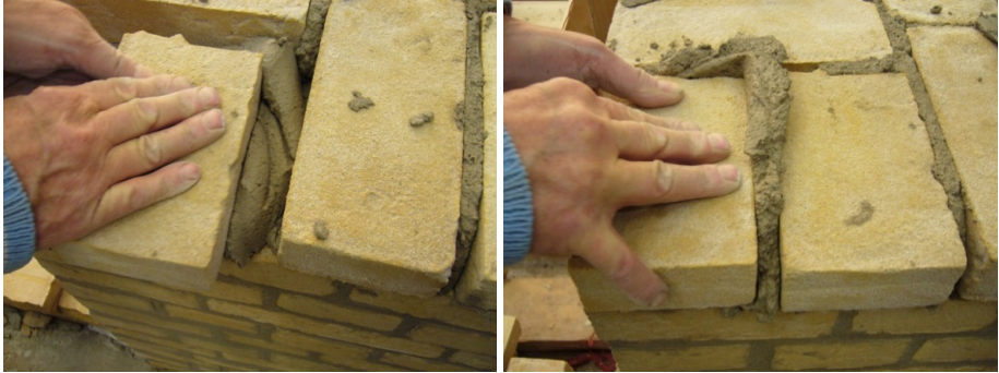
Figure 13. A basic requirement for water tightness is that during execution no voids are left; to avoid this every brick should be fully surrounded by mortar. This is only possible if the brick laying is done carefully brick-by-brick.
