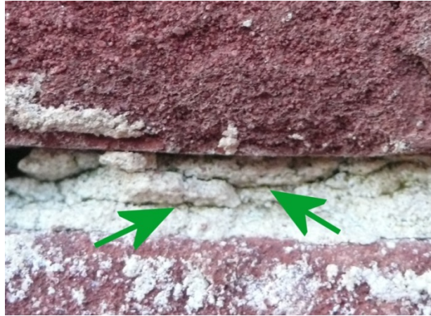
Figure 4. Frost damage in an uncarbonated air lime mortar due to an application of the mortar too late in the season (Brussels, Belgium)
