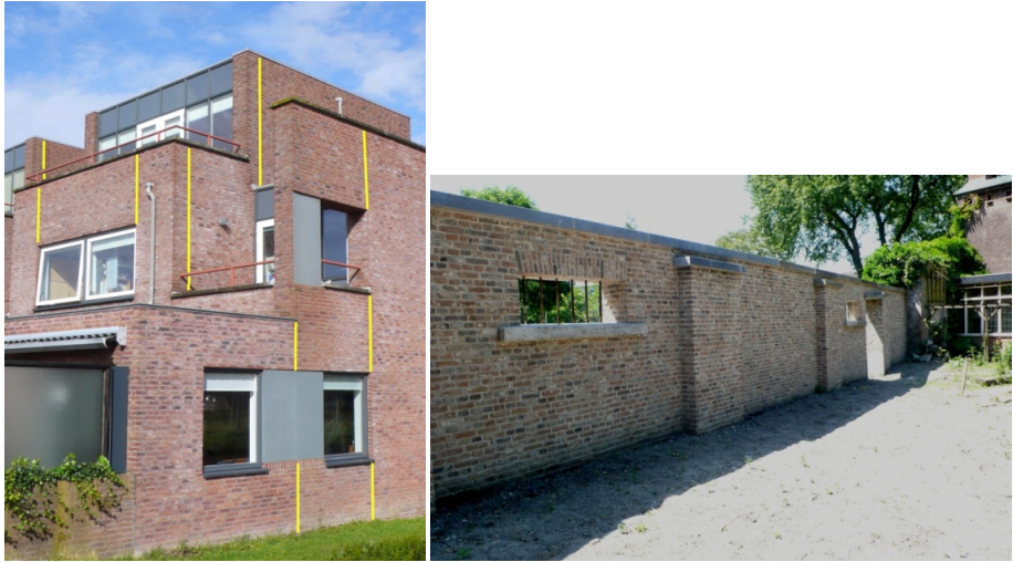
Figure 9. Left: many expansion joints in modern cement mortar masonry (see the yellow lines). Right: in this wall built with a natural hydraulic lime (NHL 3,5) only one expansion joint was applied at the top of the door opening at the rear of the wall.
