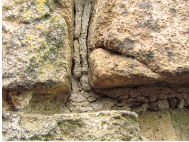
Figure 3. Frost damage of lime-based bedding mortar caused by a high degree of saturation (in West wall of Ruin De Nijenbeek, the Netherlands)
